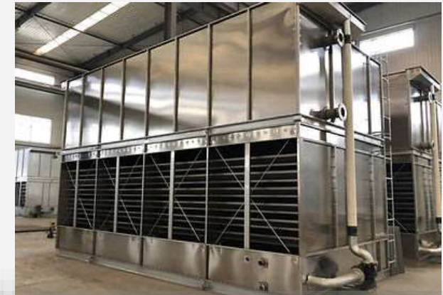
Individual air cooling units
