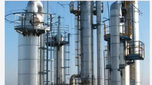
Amine purification columns for gas processing complex
