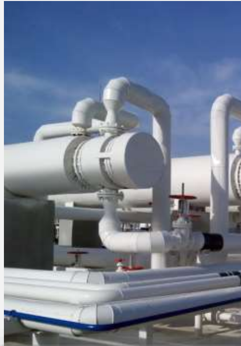
Heat exchange equipment
